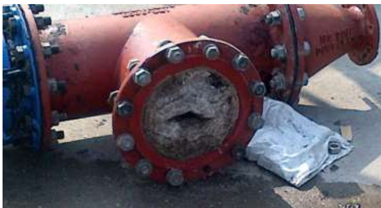
Figure 7: Problem Struvite precipitation in existing Stoke Bardolph liquor pipework
